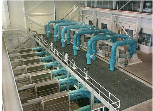
FIGURE 4: CORNELL UNIVERSITY LSDC HEAT EXCHANGE FACILITY 4
