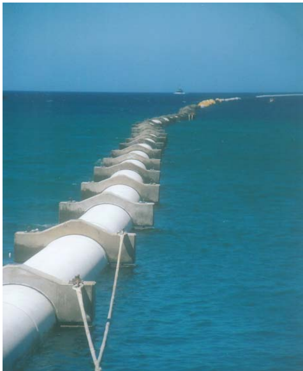
FIGURE 3: COLD WATER PIPE DURING DEPLOYMENT 8
